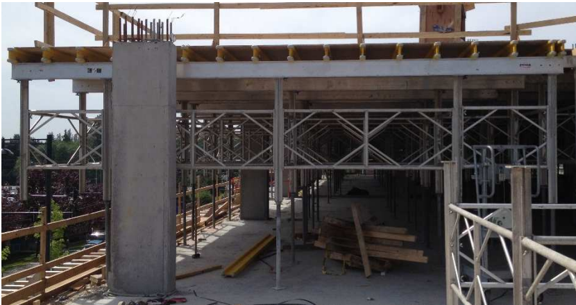
Cantilevered tables with HV extension
